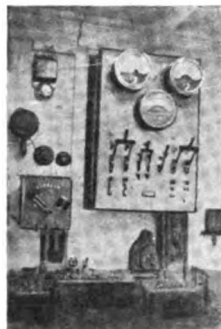
Starting box and power panel for main 3 kw. set
