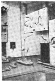
Loading coil panel and antenna switch
